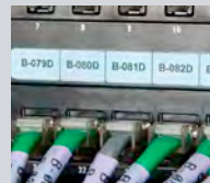
Patch Panel & Terminal Block ID
